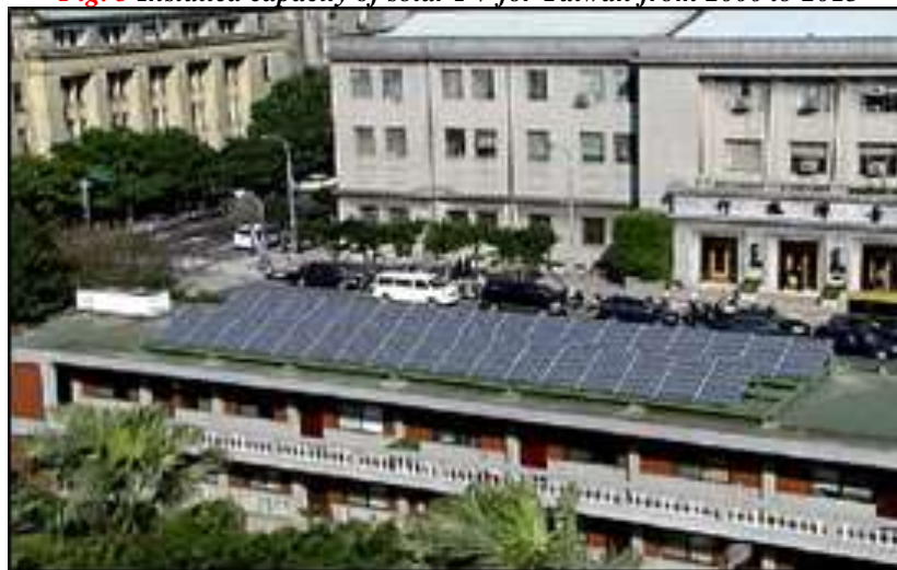
Fig. 6 Presidential Hall demonstration system (10.5 kW)
